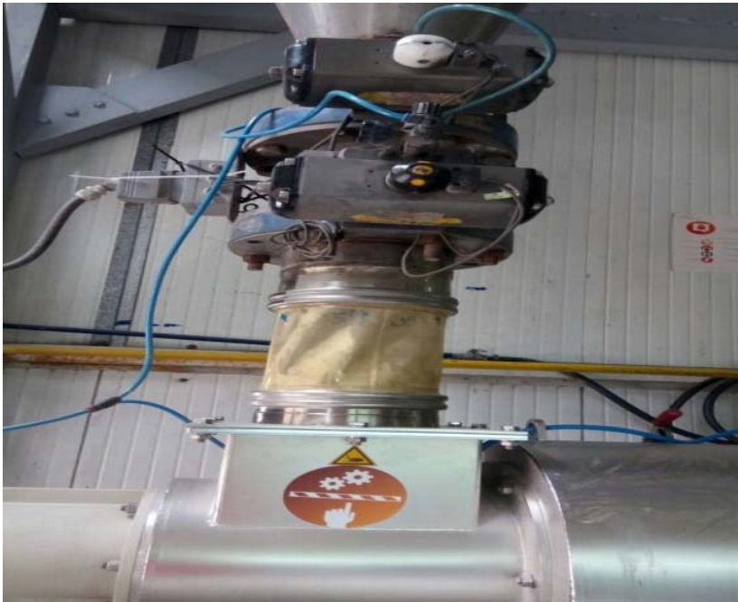
On site Double Flap Gate Valve
